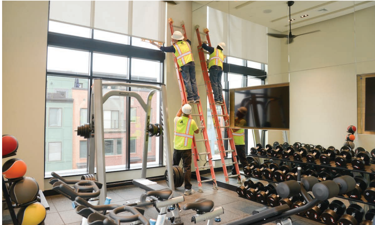
Installers from CIP Finishes hang motorized blinds in a fitness center at the second phase of the Modera Mosaic apartments in Fairfax County's Mosaic District.
